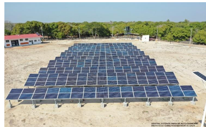
Central Solar de Alto Changane (100kW)-Gaza
